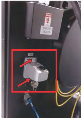
J33 terminal block 1 shown here with the location of the mounting screws indicated with the red arrows
